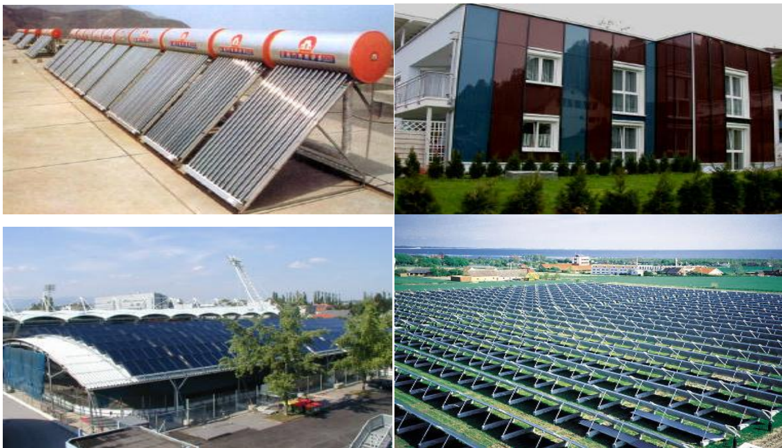
Figure 2: Solar Thermal Systems in Operation in DCs
